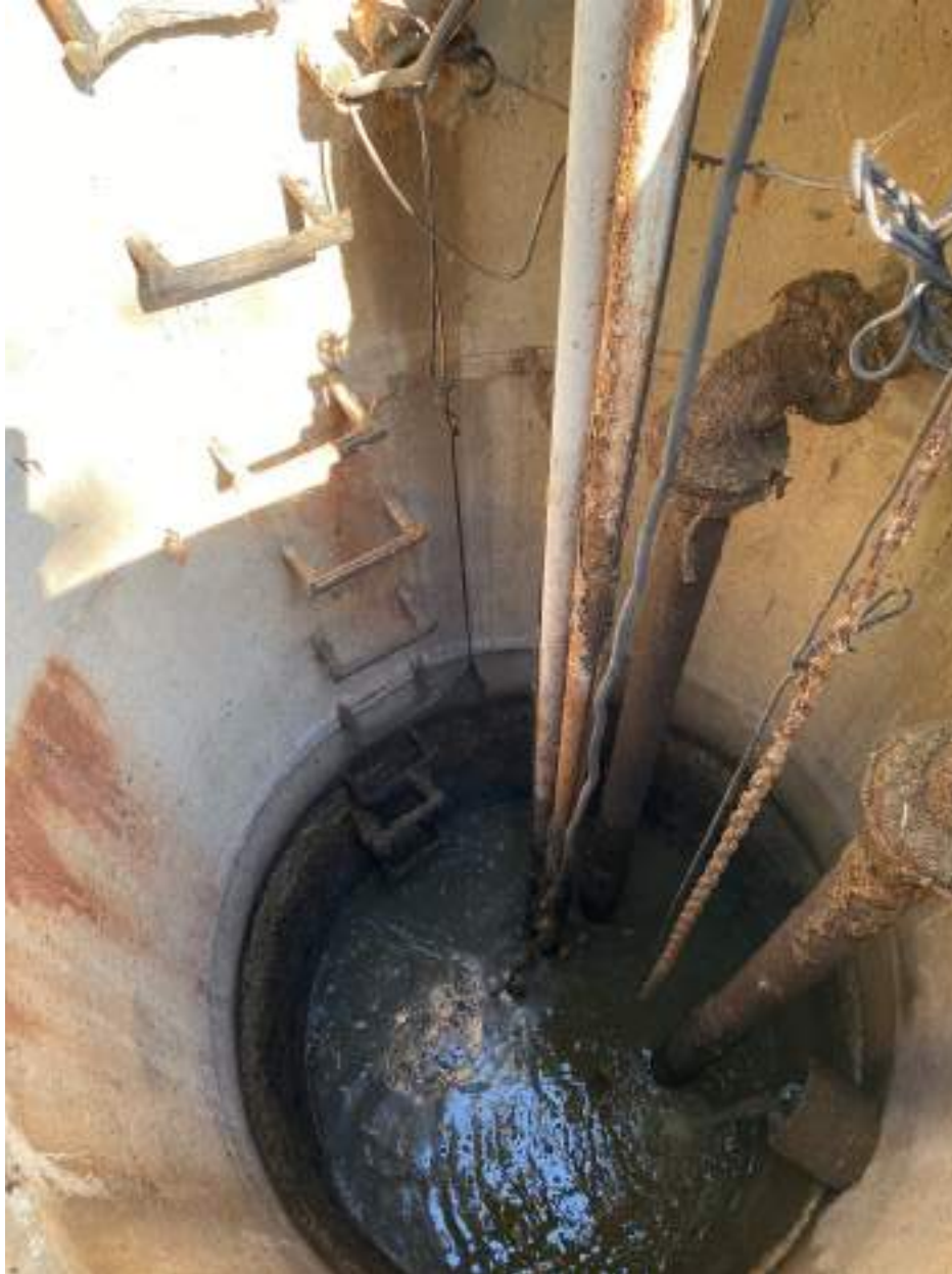
Photo 8 Wet Well No. 3 – Note Single pump and missing guide rails
