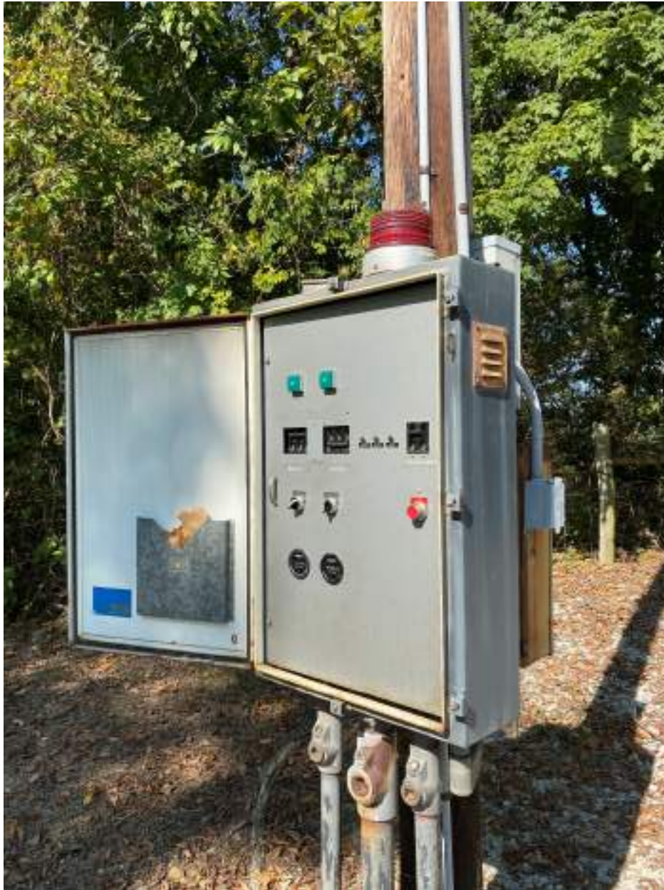
Photo 12 Electrical No. 3 – Control Panel Opened
