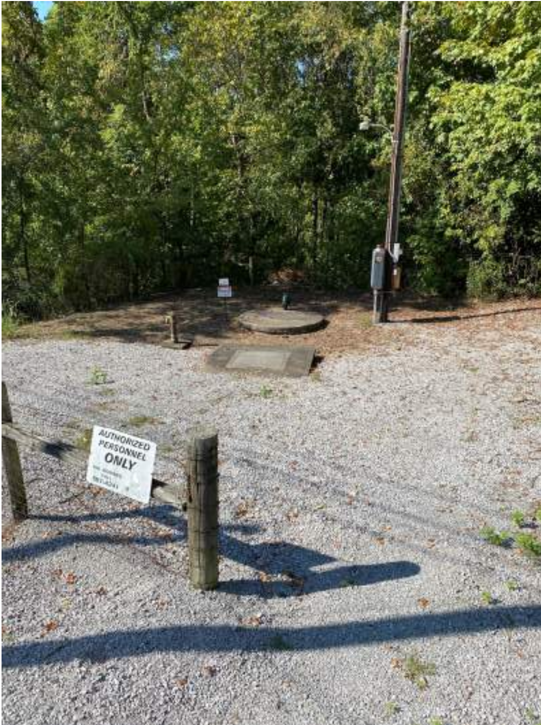
Photo 1 Site with Gate, Wet Well, Valve Vault, Power Source, and Yard Hydrant
