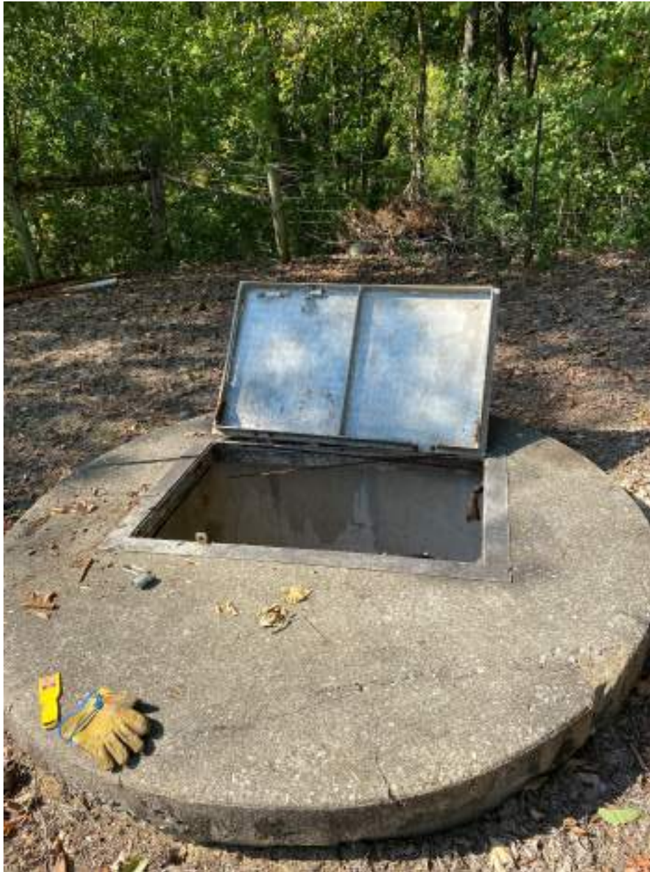
Photo 6 Wet Well No. 1 – Note broken hinge
