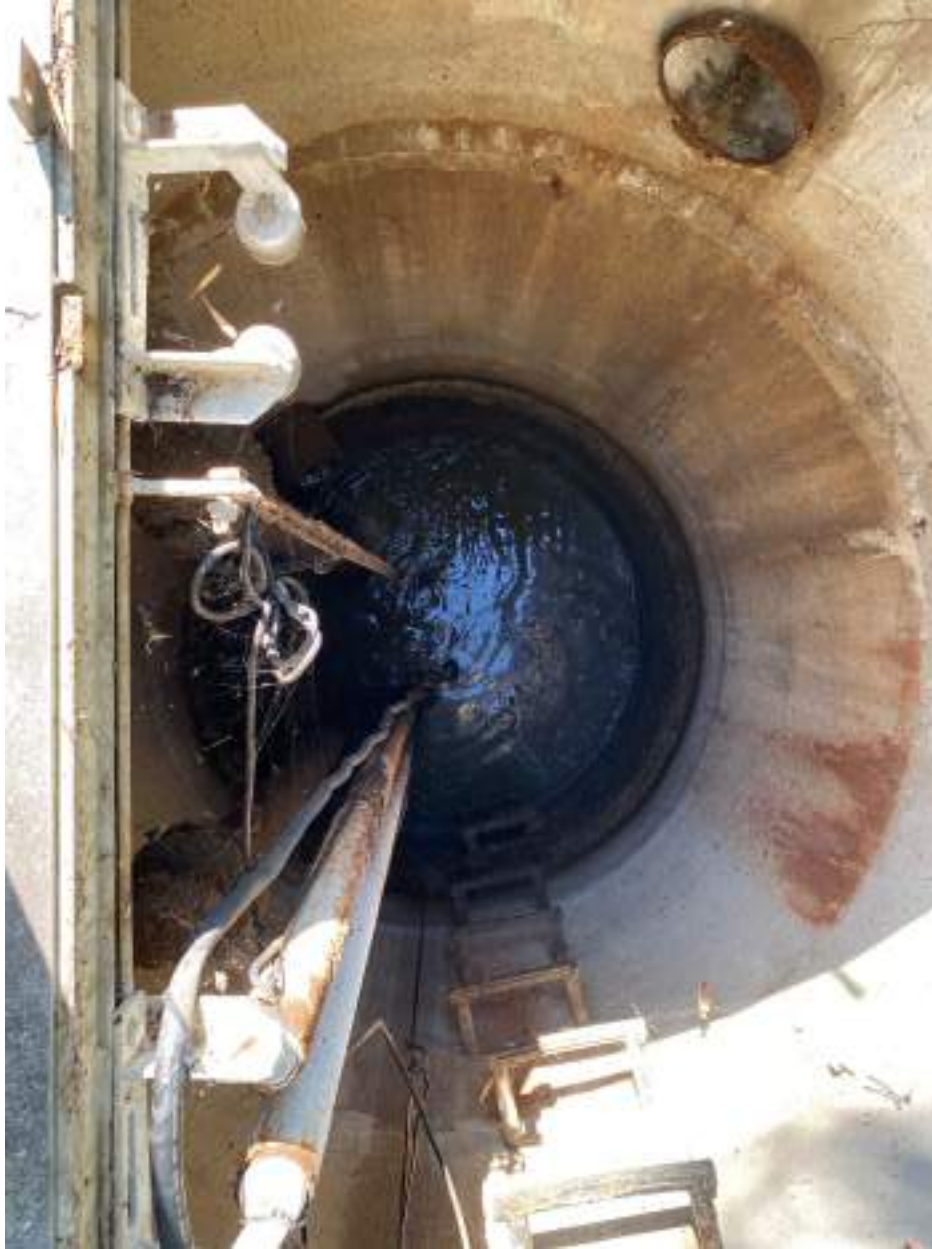
Photo 7 Wet Well No. 2 – Note Single pump and missing guide rails
