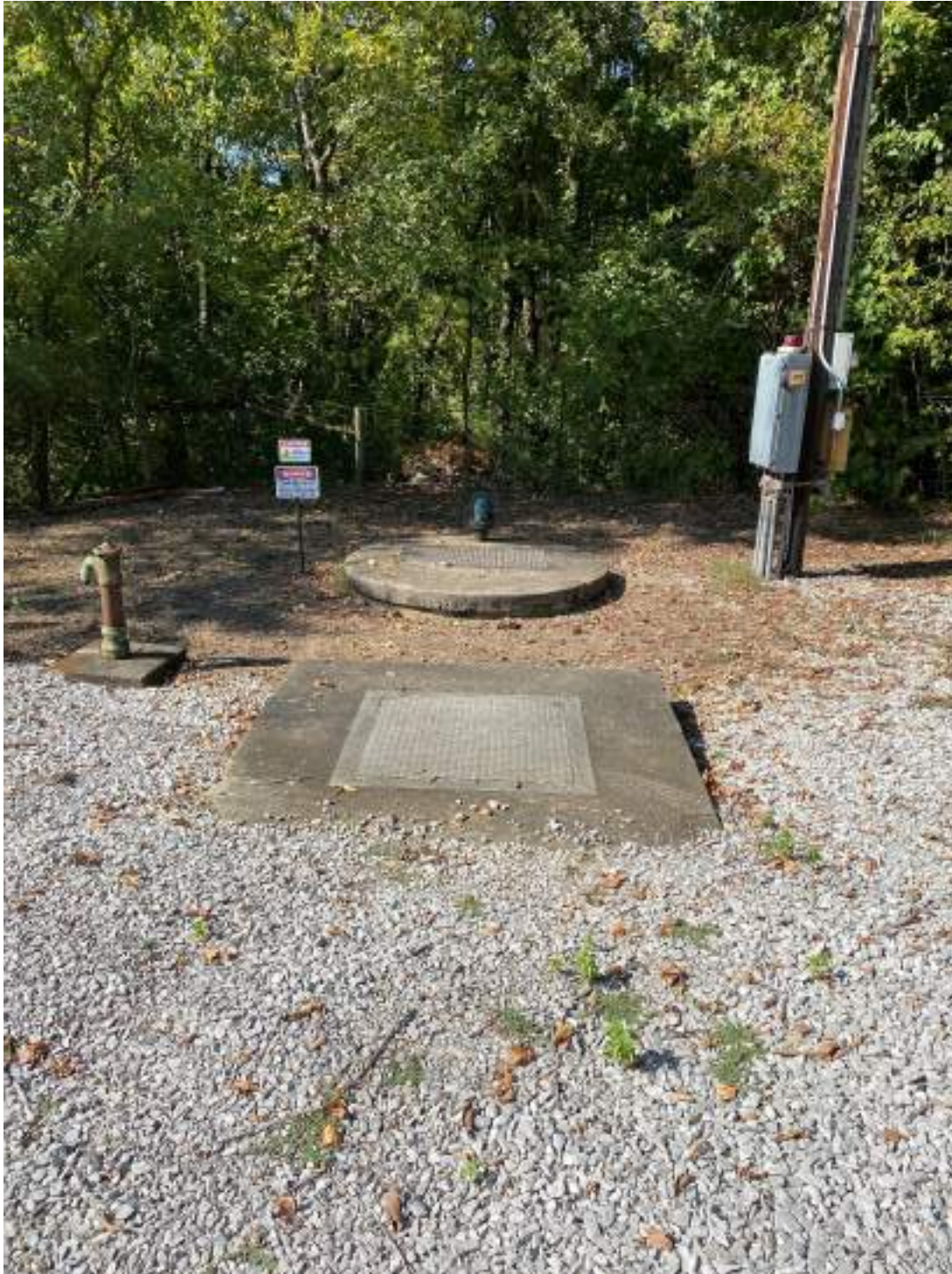
Photo 2 Site with Wet Well, Valve Vault, Power Source, and Yard Hydrant
