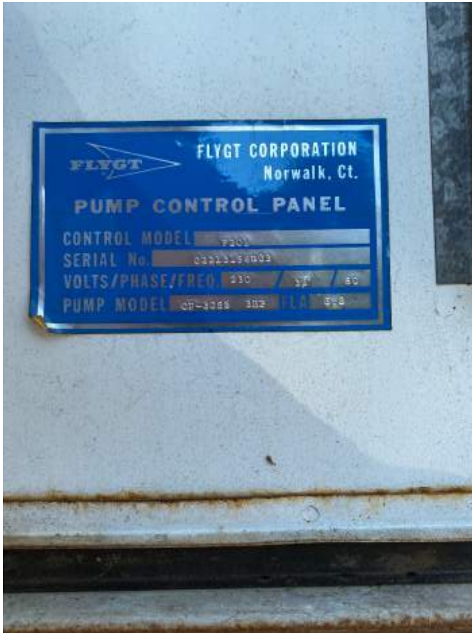
Photo 11 Electrical No. 2 – Control Panel Factory Decal
