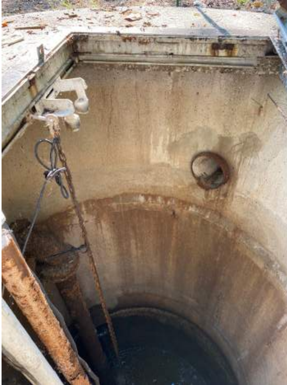
Photo 9 Wet Well No. 4 – Overflow pipe to be plugged
